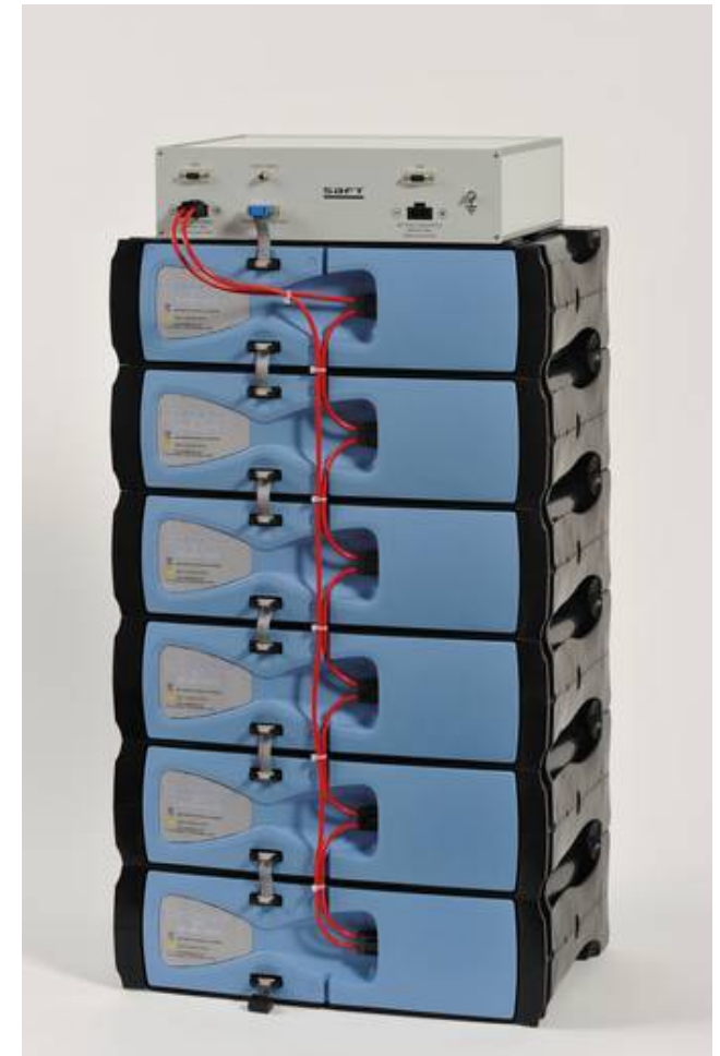
Example of battery system 288V, 13kWh
