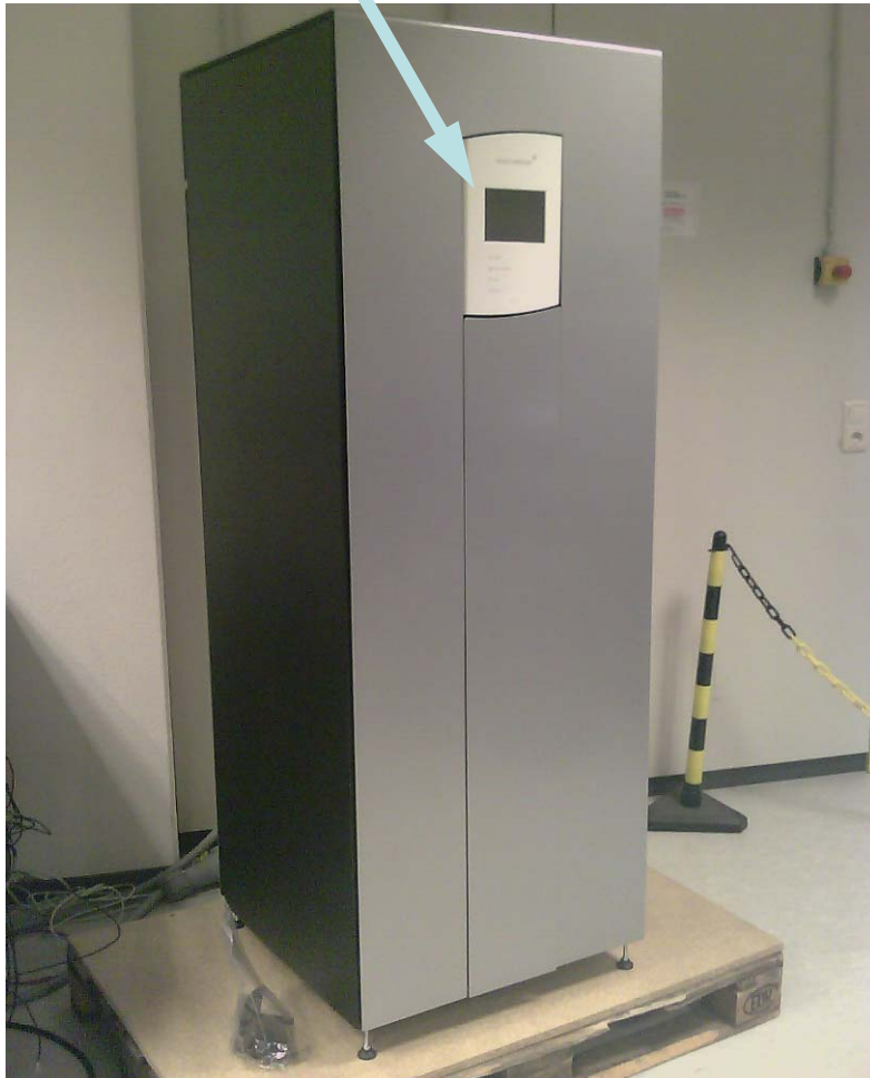
Energy Management System
